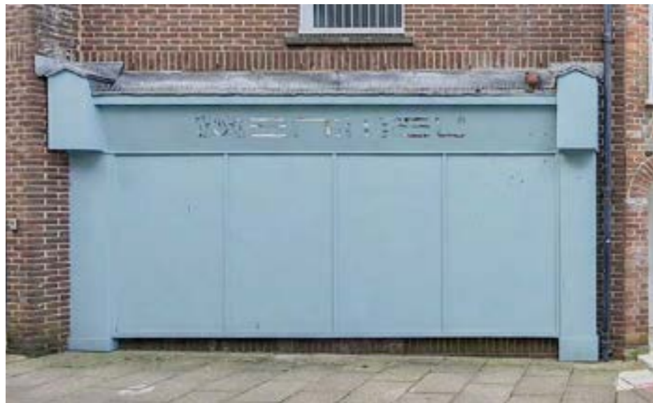
Simplified modern recreation of traditional shopfront framing using pilasters, consoles and fascias, to the rear of no. 34
