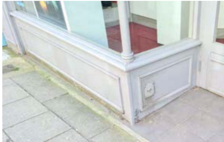
Existing shop fronts currently exhibit references to traditional detailing that should be re-implemented in a higher-quality and more coherent manner suitable for contemporary shop fronts
