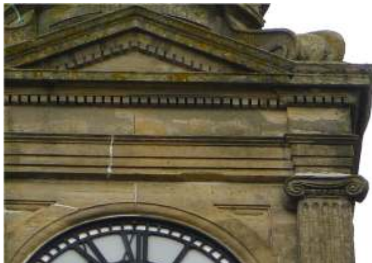
Figure 6: Photo [2021] repointed cracking to west face of the clock tower - which has not re-opened
