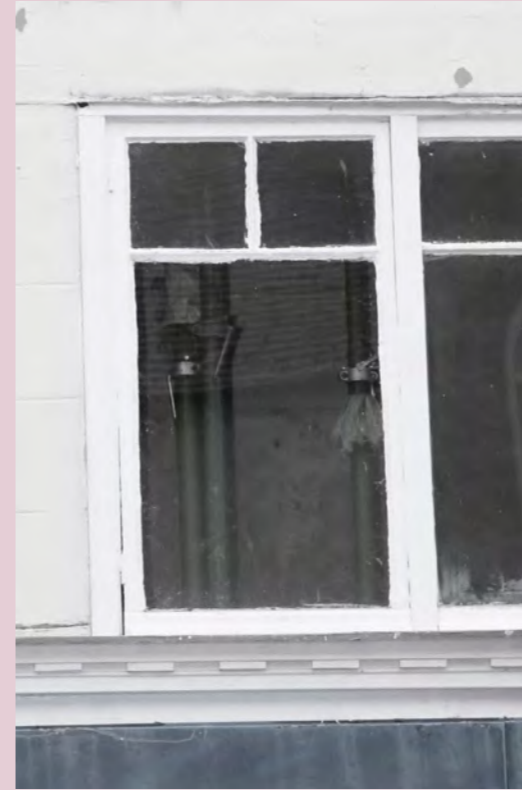
Above: An “acrow” temporary structural support visible through a first floor window, implies that not only is the first floor not in use but that the building requires important maintenance.
