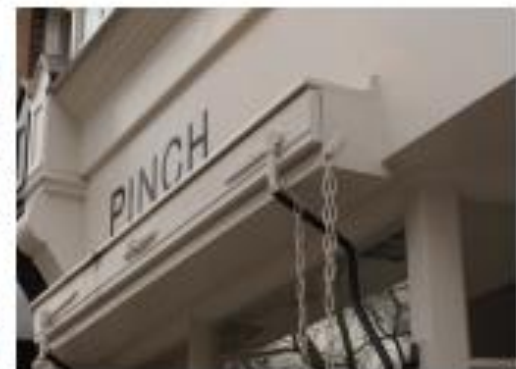
A good example of a blind that is not integrated into shopfront, London
