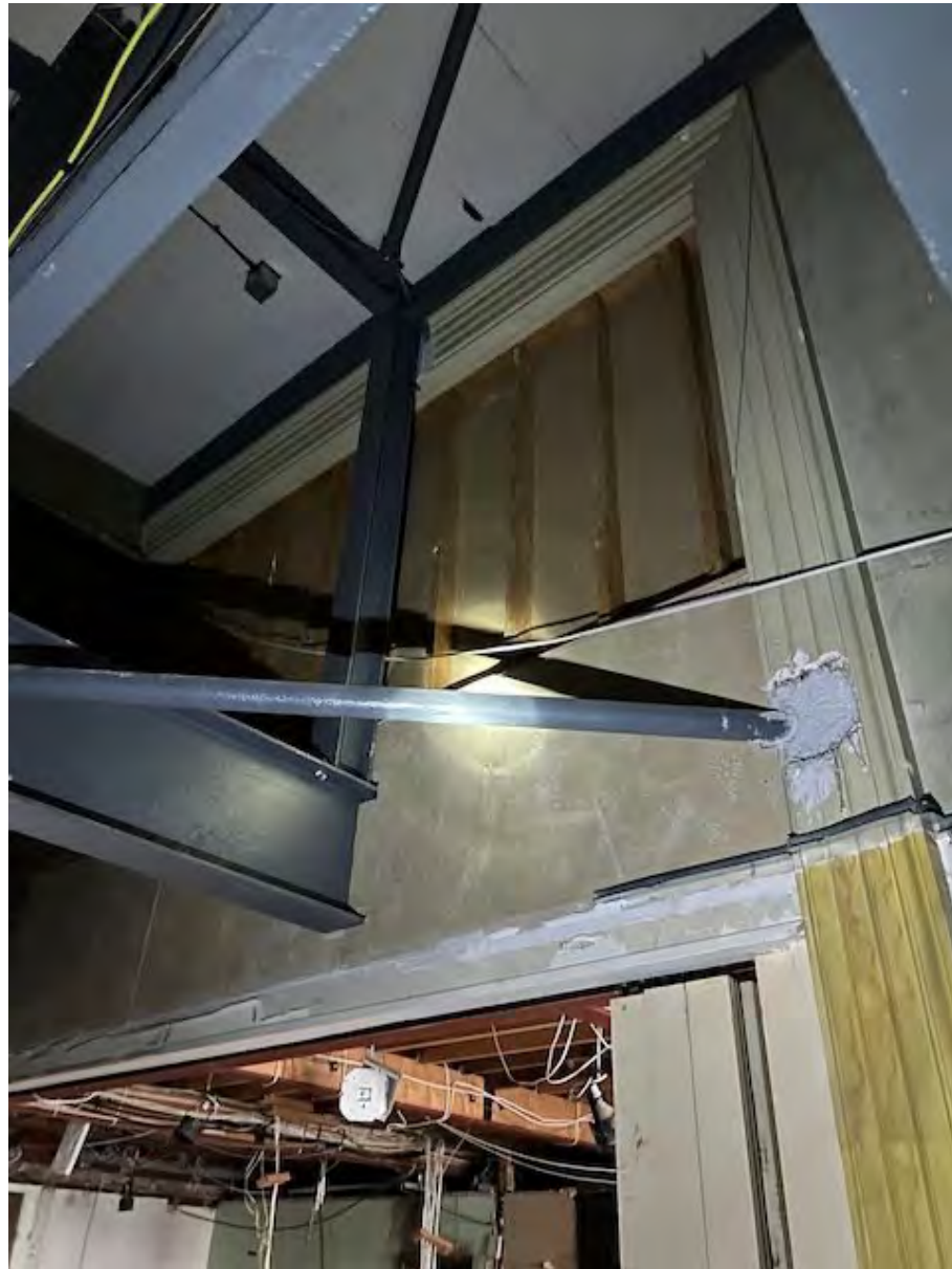
Steelwork cut through moulded plasterwork
