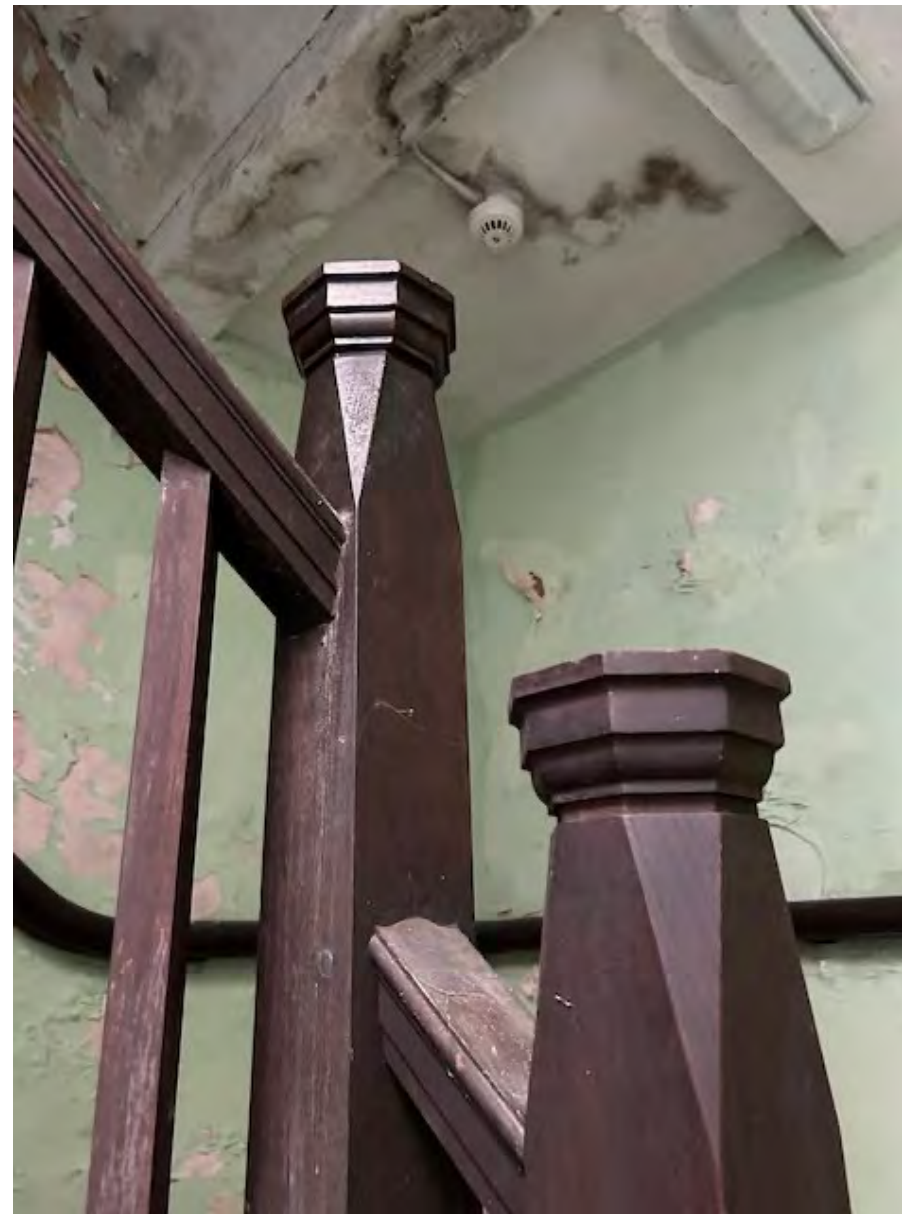
1930's stairs following the fire (oak)
