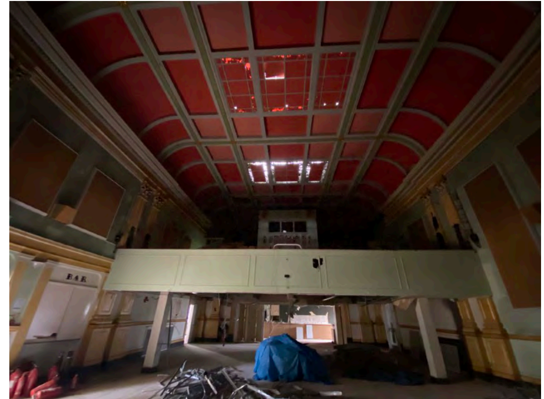
Modern Balcony inserting in 1990. Note painting over former glazed openings at roof level
