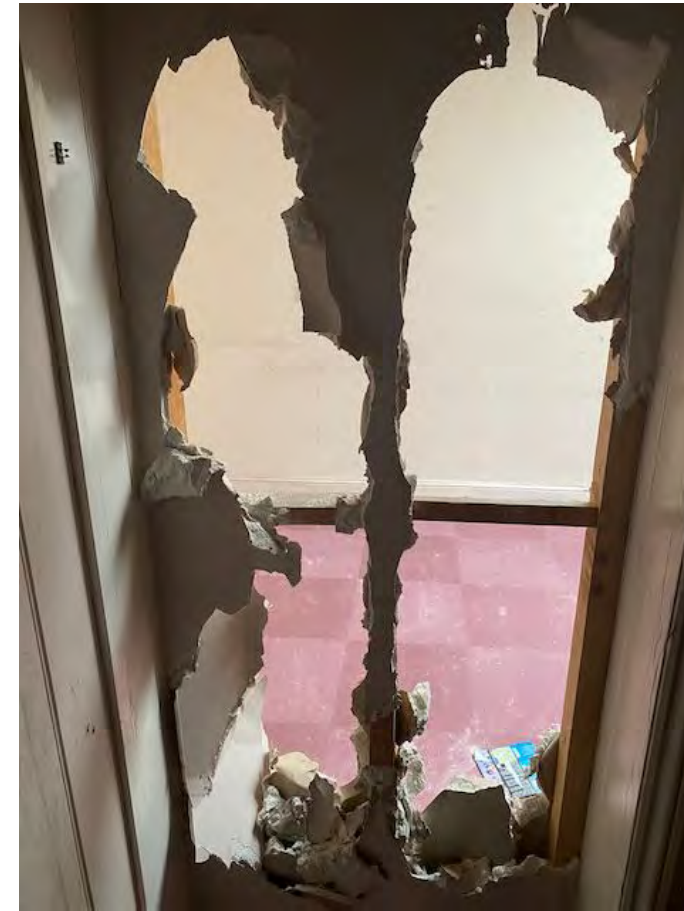
Deliberate damage to internal building fabric
