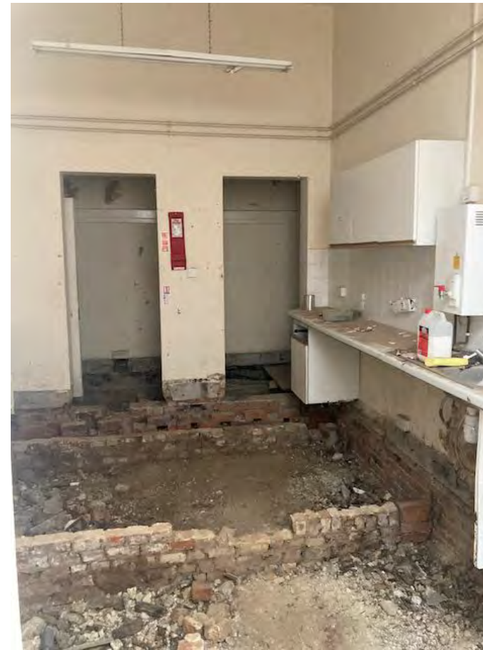
Missing floor and redundant kitchen units (believed to be the origin of the dry rot infestation).
