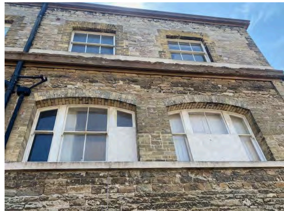
Damaged string course. Note change of masonry 3 courses below rendered string course. Lower sections original, with extension above.
