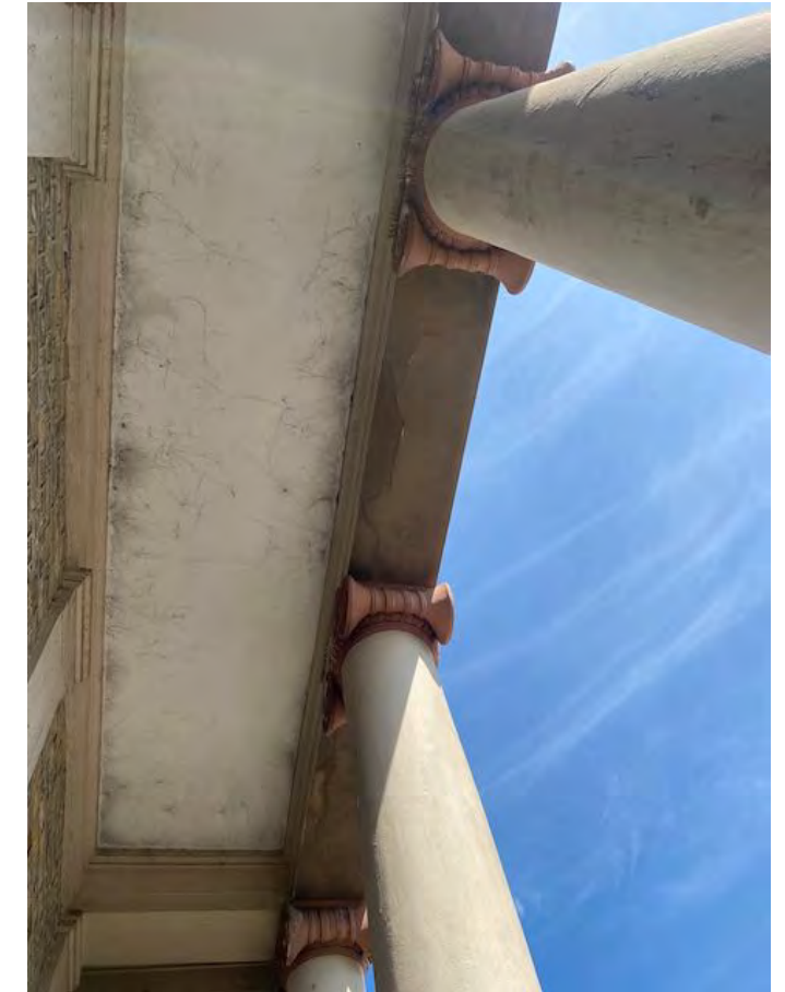
The column capitals with the painted volutes. Note cracking to underside. Corrosion to steelwork above
