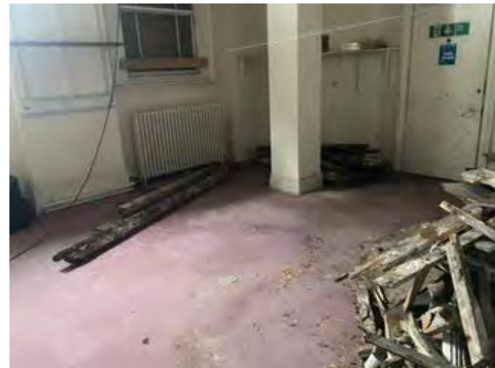
Infected timber and fire escape door
