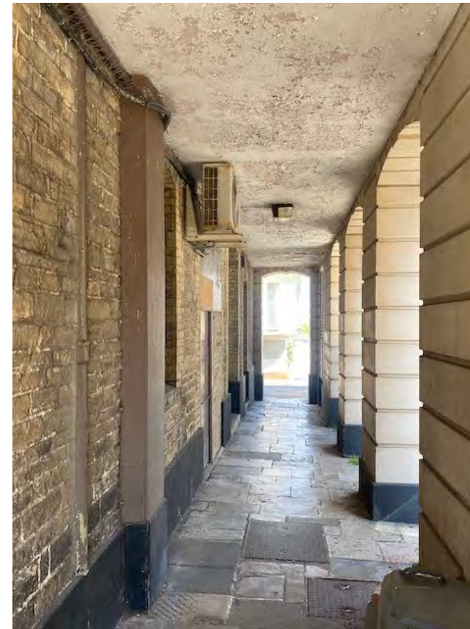
Downpipe embedded in the wall of the east end of the building. (left of picture). Entrances to public toilets
