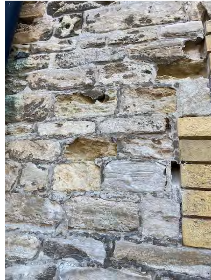
Badly eroded stone as a result of masonry bee attack
