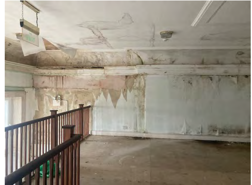
Penetrating damp upper part of bar (mezzanine)
