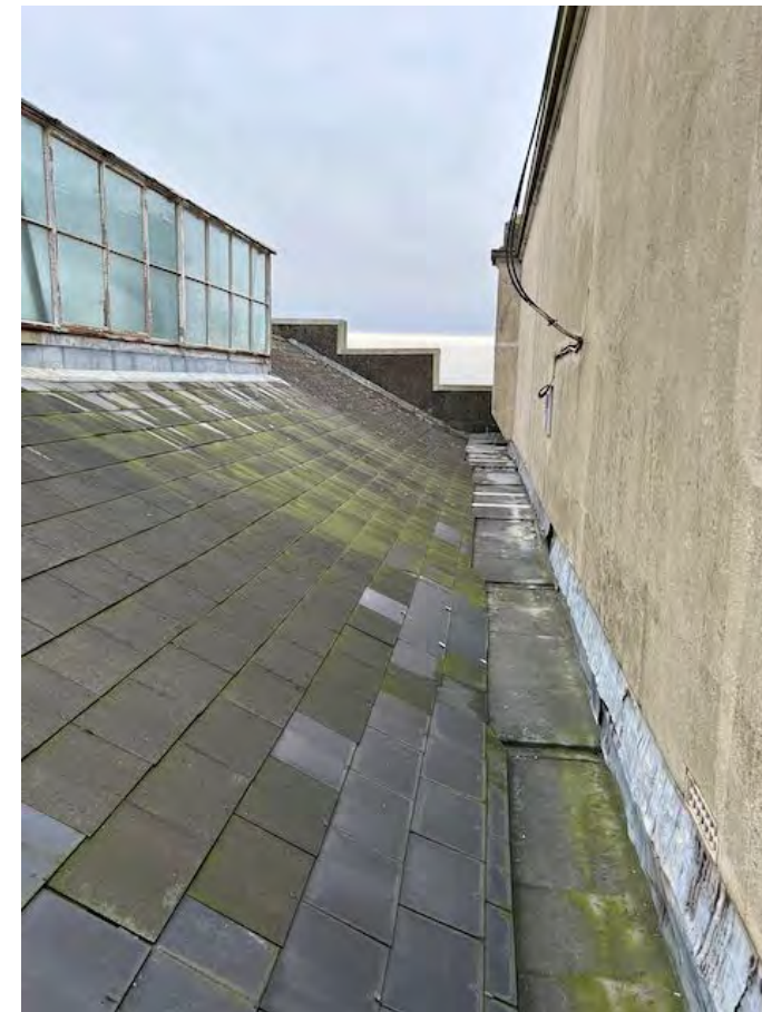
Cracked lead in valley gutters causing
