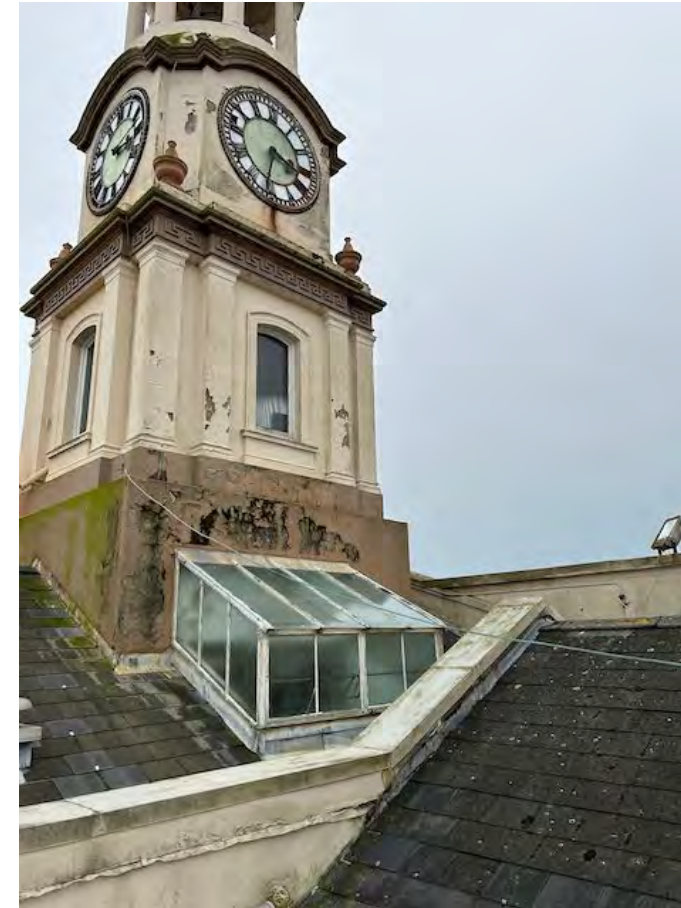
The Clocktower from the North west. Extensive cement repairs
