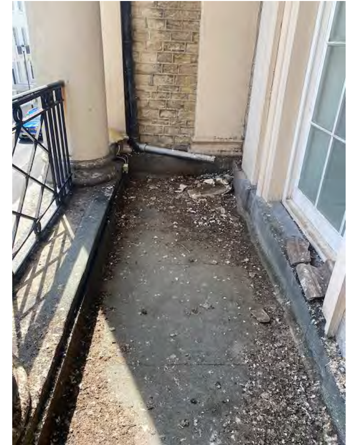
Balcony surface showing pigeon droppings
