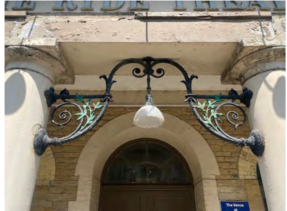
Decorative wrought iron light fitting
