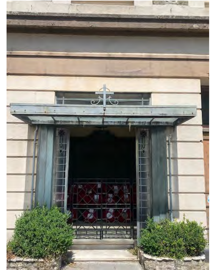
Vertical cracks in render above the war memorial.
