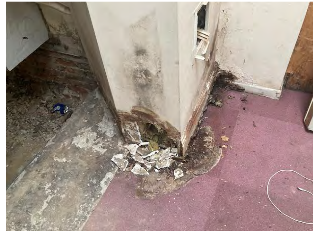
Damaged drainage chamber and dry rot fungus
