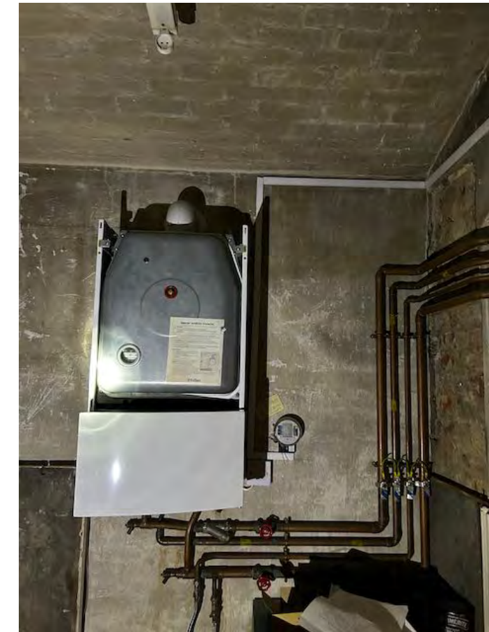
'Modern' Gas boiler to west range. Pipework fair.
