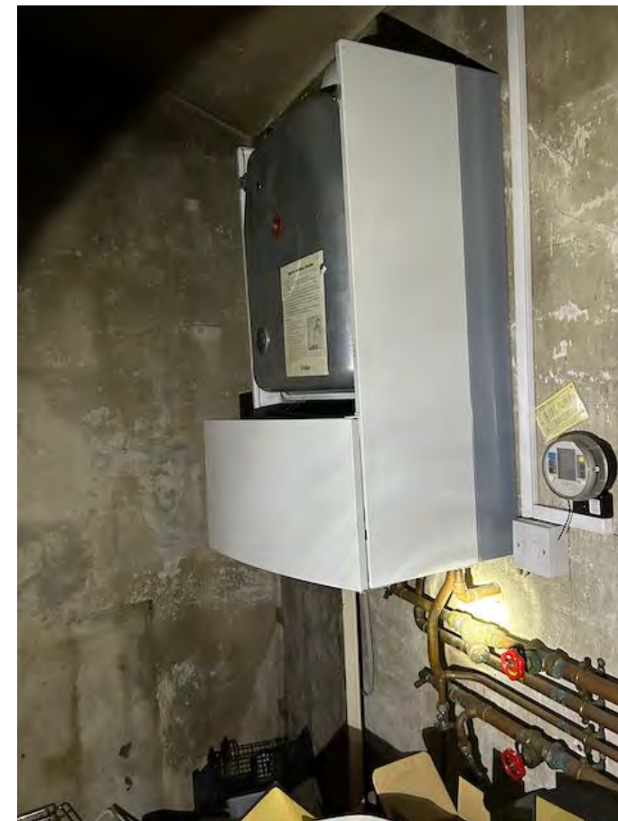
One of the boilers found within the building
