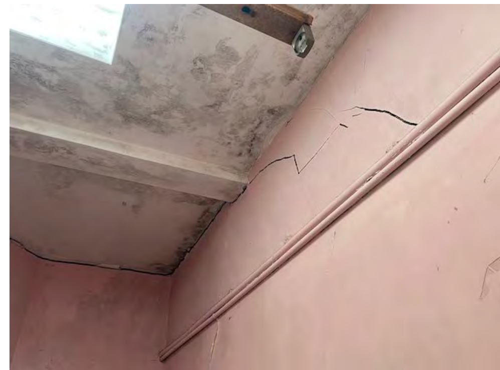
Structural movement evident within the building
