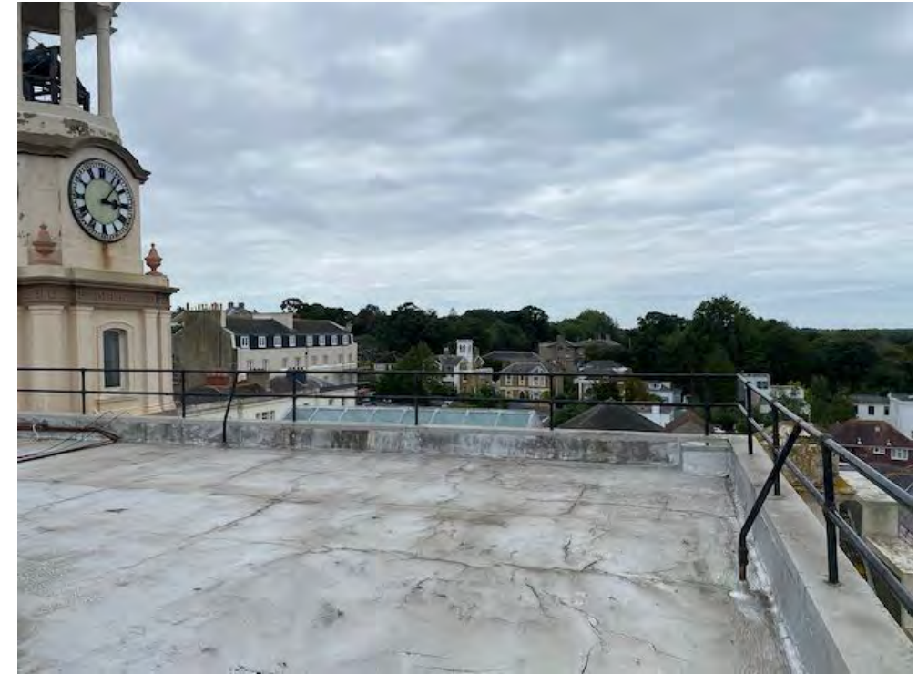
Cracked asphalt roof covering above the auditorium
