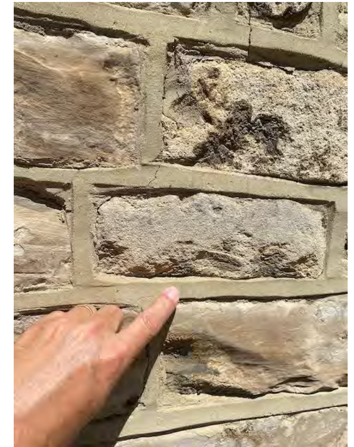
Cementitious Ribbon pointing
