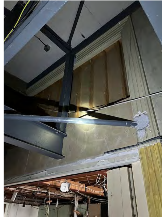
1990's insertions and damage to 1930's fabric
