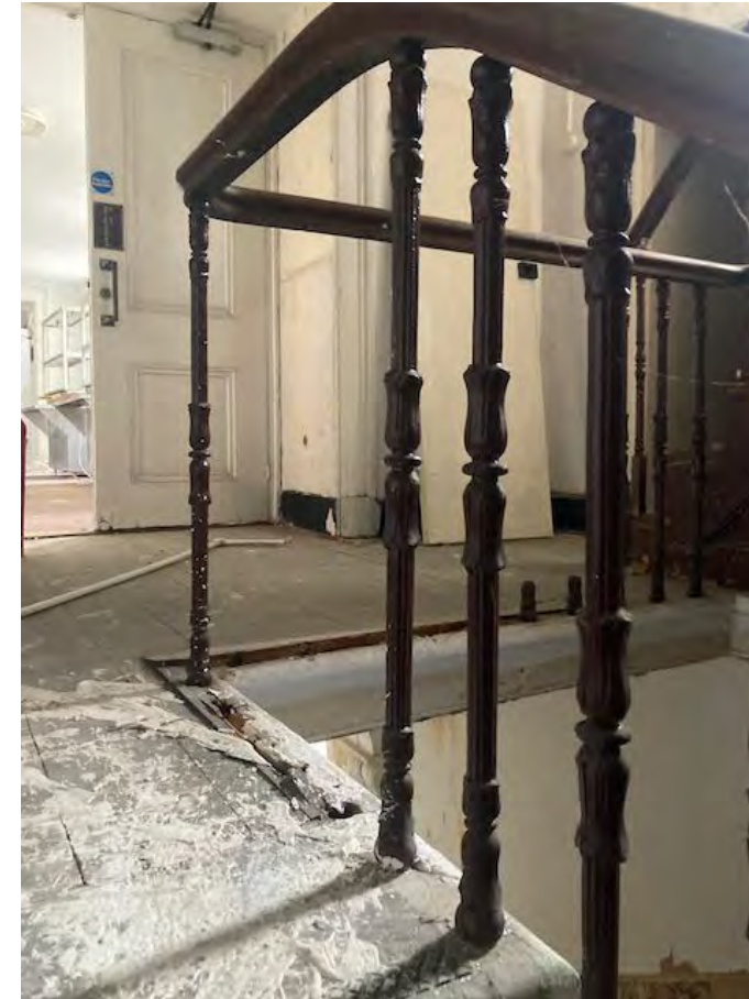
Broken spindles on staircase
