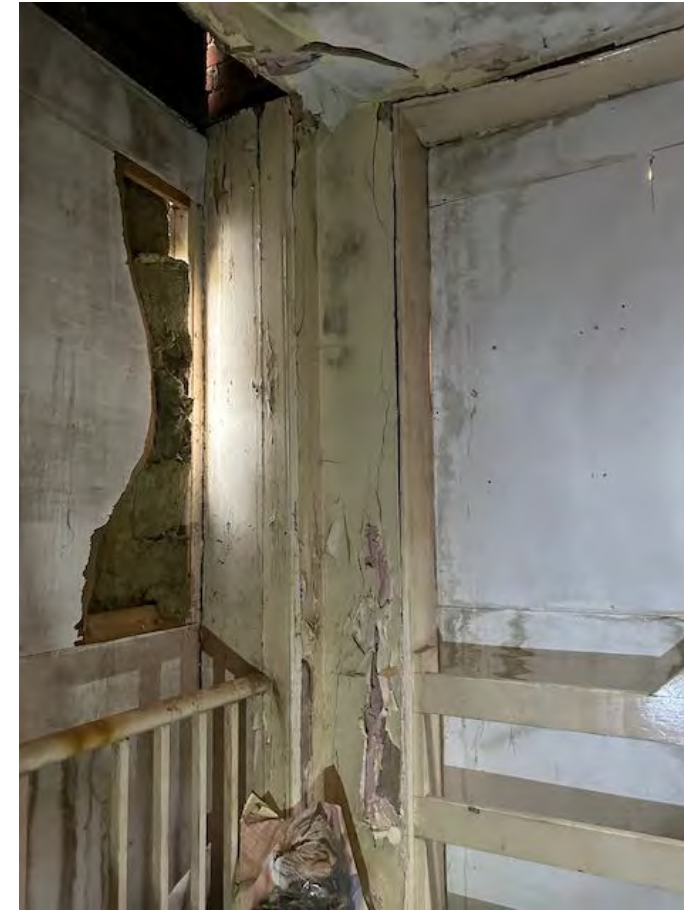
Extensive cracking to SE corner. Note close proximity of openings to the corner (south and east walls) which is a potential source of weakness.
