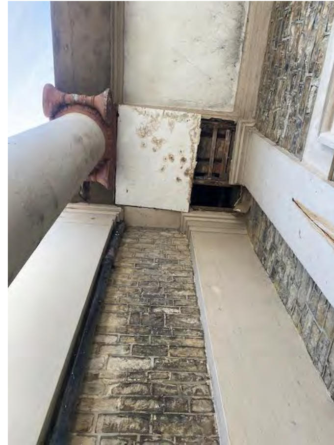
Section of failed ceiling exposing timber joists. Note wrought iron spanning between column and south elevation of building
