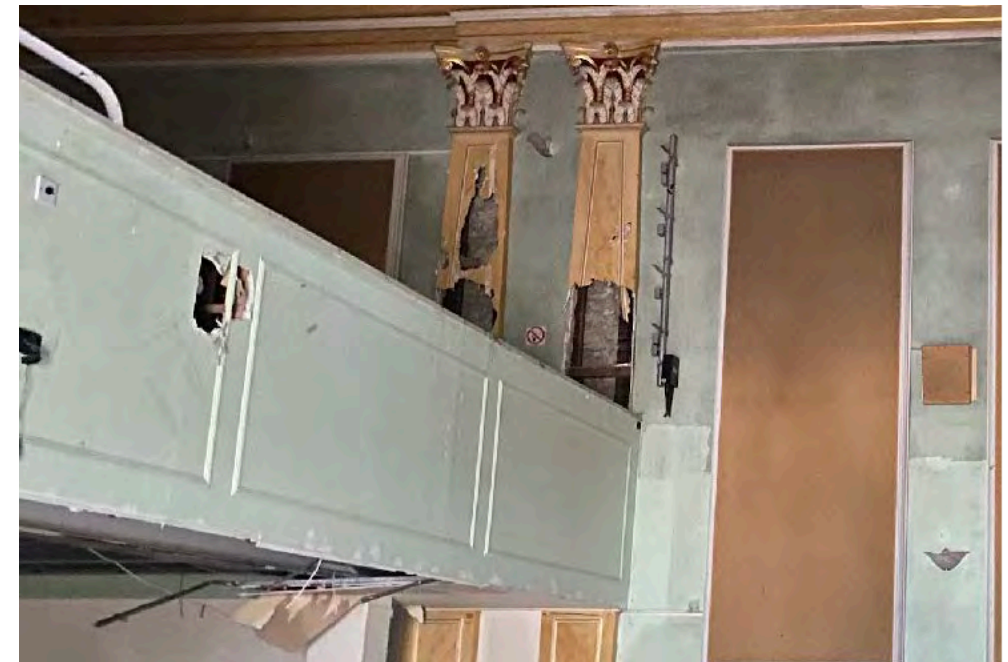
Damaged pilasters at balcony level
