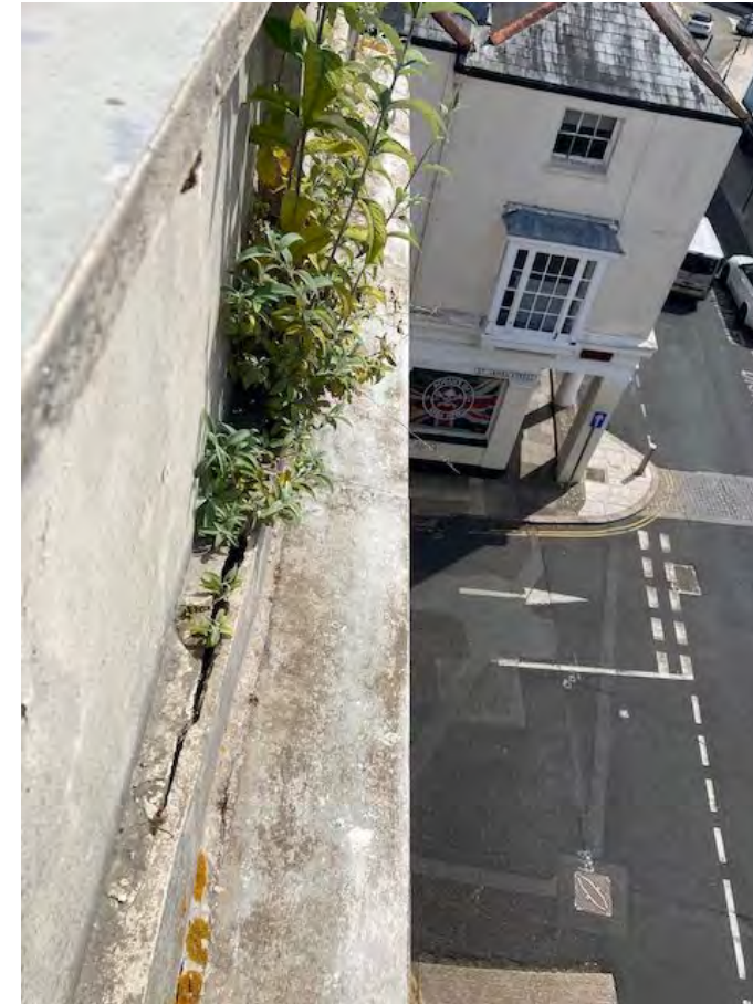
Buddleia forcing coving away from southern elevation
