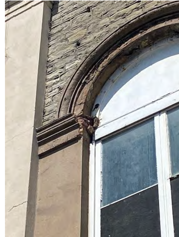
Significant decay to the run moulded cornice
