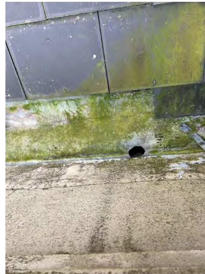
Hole in lead gutter. Urgent repair required
