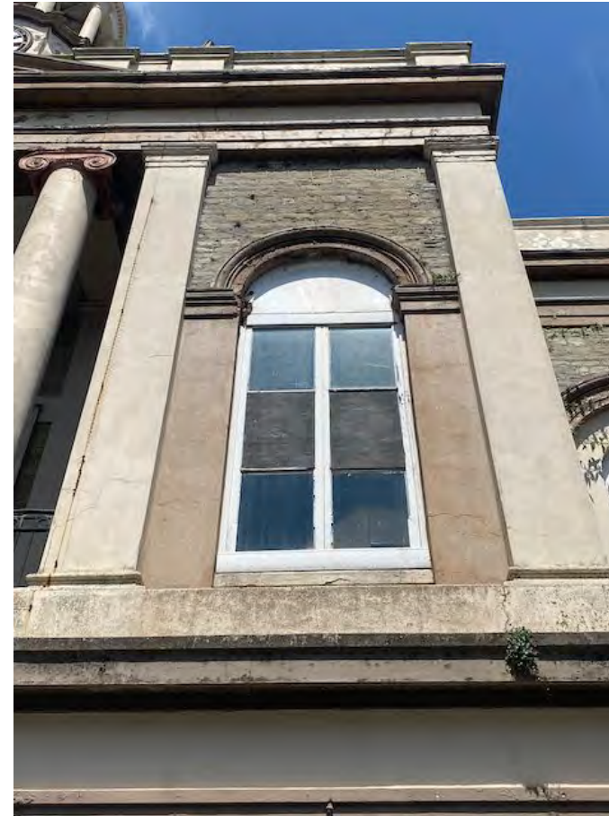
Horizontal cracks through the render of the eastern pilasters
