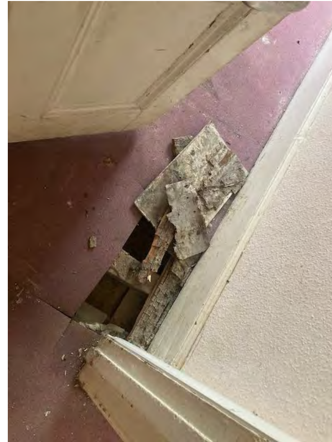
Floor boards and floor joists damaged by dry rot (G18)
