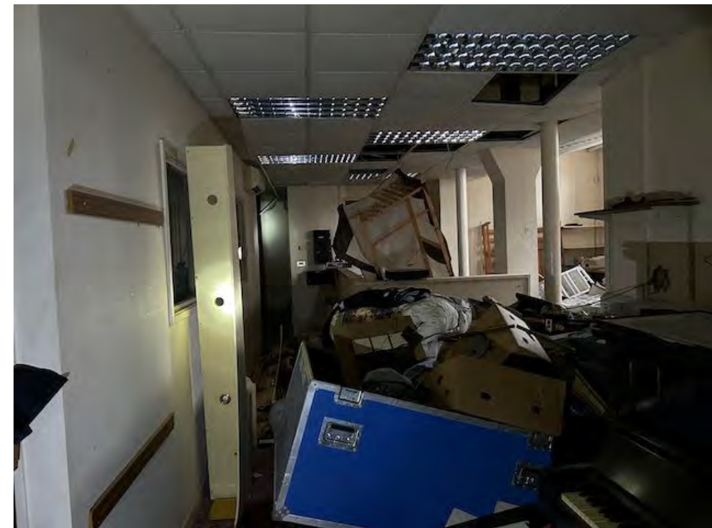
Extensive clearance of areas of the building required.
