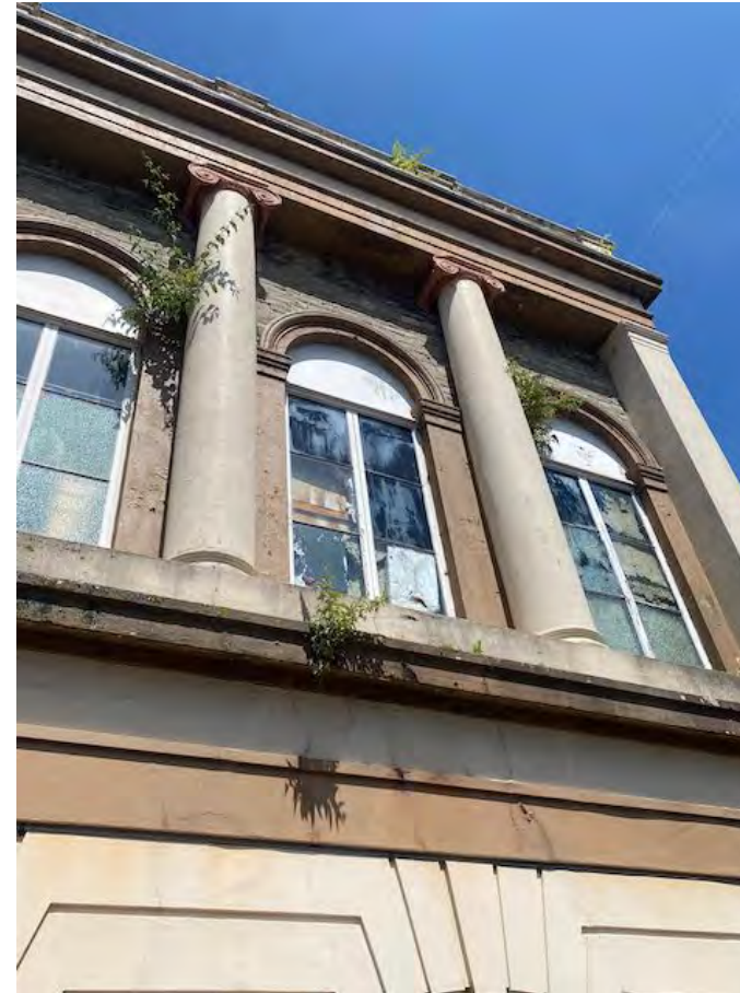
Areas of established Buddleia on the eastern pavilion
