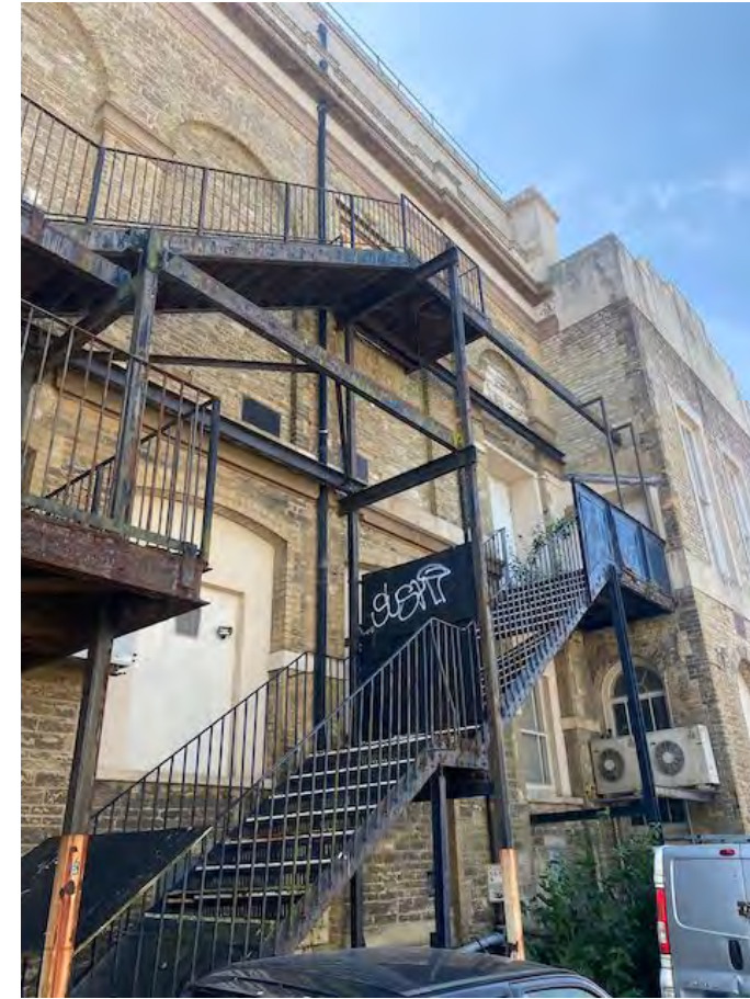
Fire escape on the north elevation. Urgent works required.
