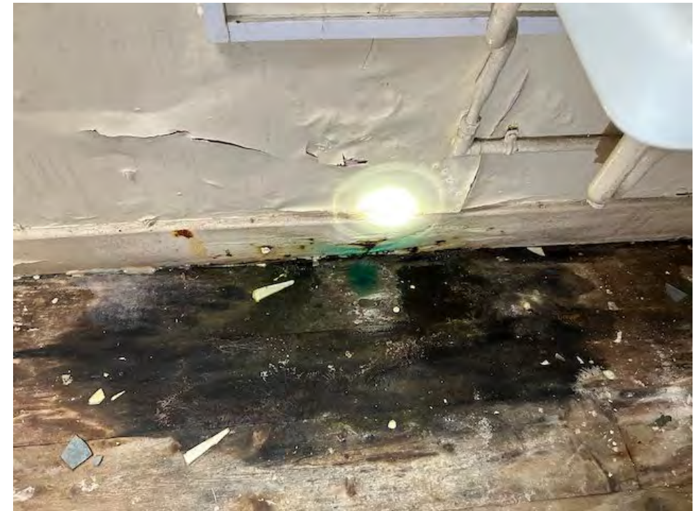
Very damp floor beneath active water leak in changing rooms, increasing risk of dry rot.
