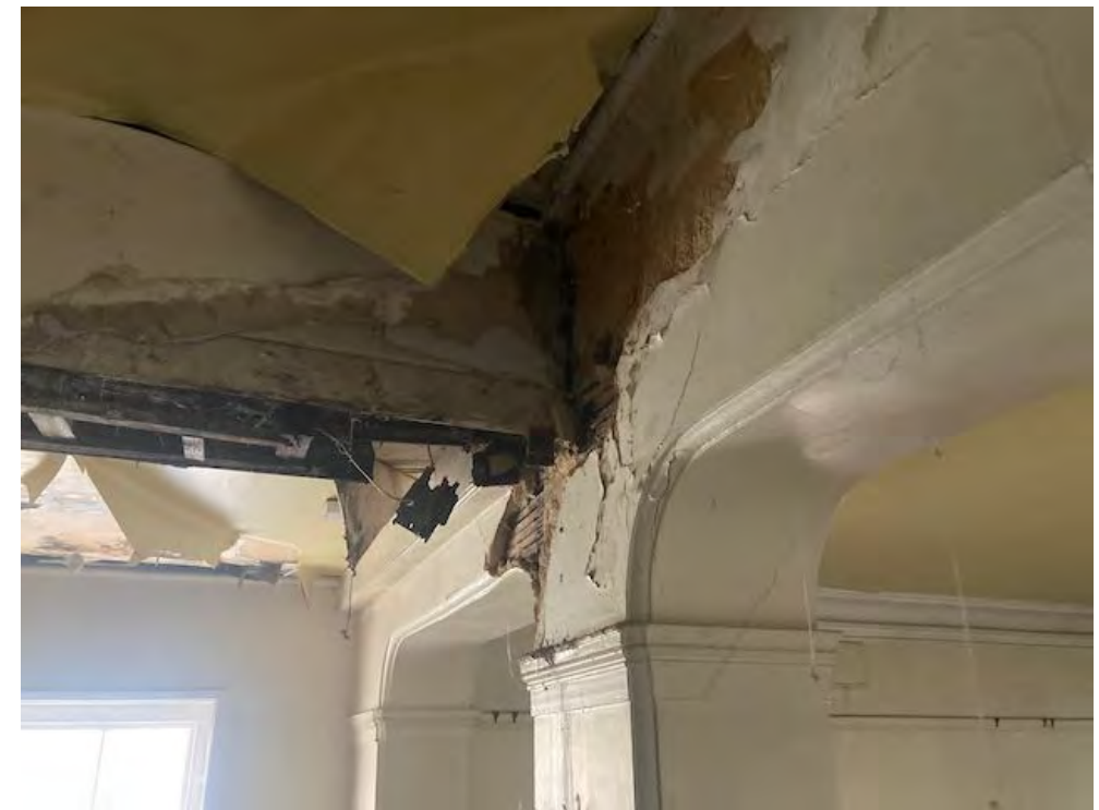
Decay to beam urgently requiring support (Urgent)
