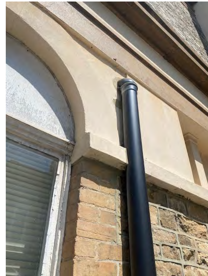
Plastic rainwater pipe penetrating the wall.
