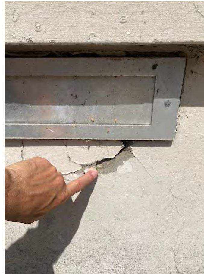
Impact damage around letter box
