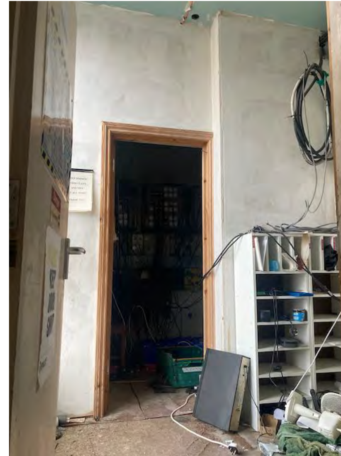
The dimmer room
