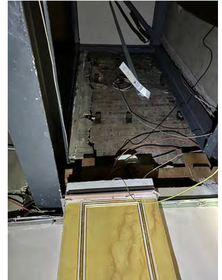
Modern plasterboard pilaster strips below balcony c.f 1930's Plaster of Paris originals
