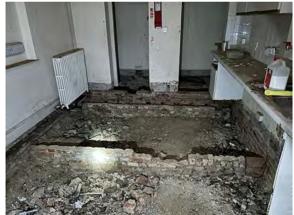
Expected original location of dry rot with contaminated material moved to G40
