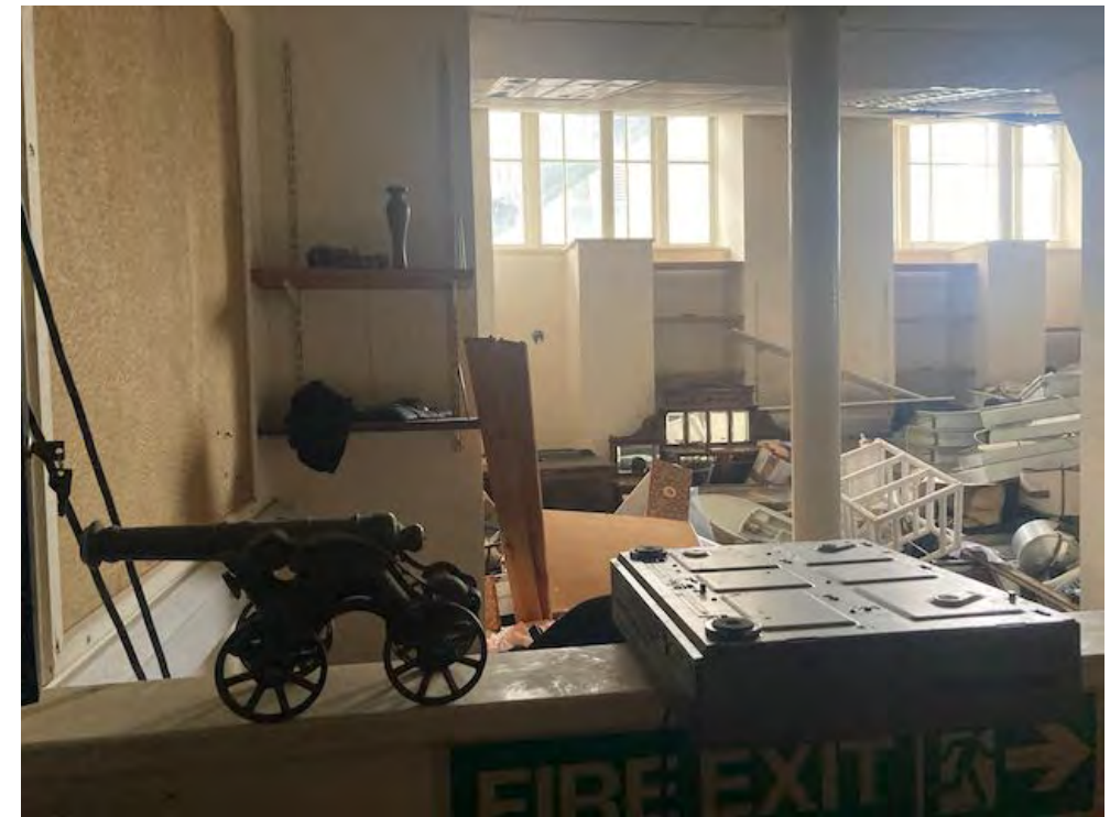
Cast iron columns providing support to the floors above. Columns shown on 1860 town plan, as subdivisions to market stalls.
