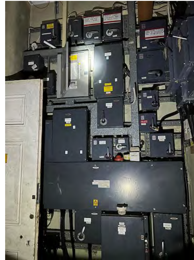
Electrical plant room
