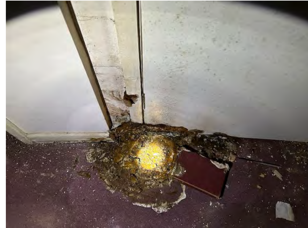
Active dry rot infestation now visible above the floor. The concealed area of decay will be very significantly larger.
