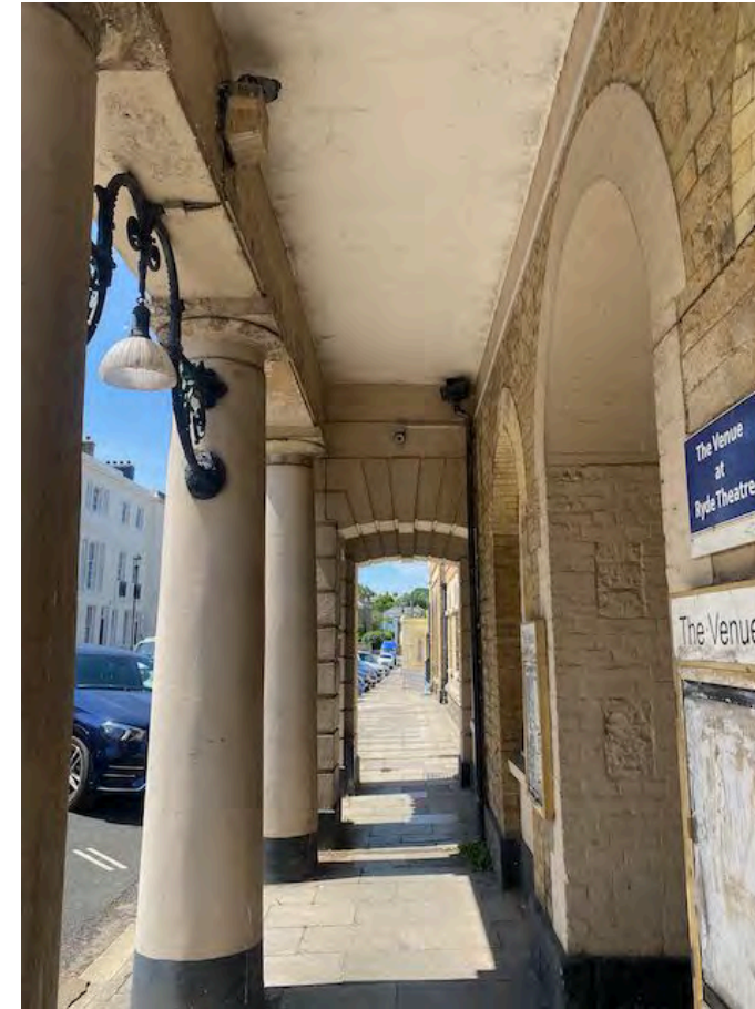
The underside of the balcony showing the display boards and the suspected asbestos soffit
