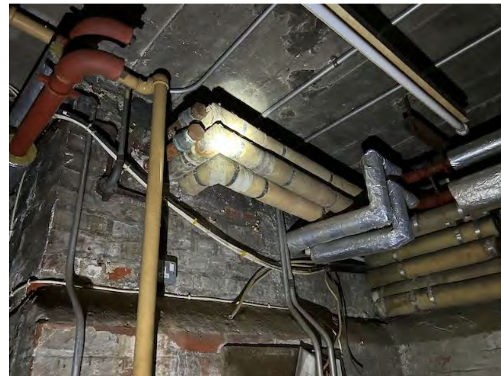
Pipework showing different phases of work and concrete soffit to ceiling. Risk of asbestos
