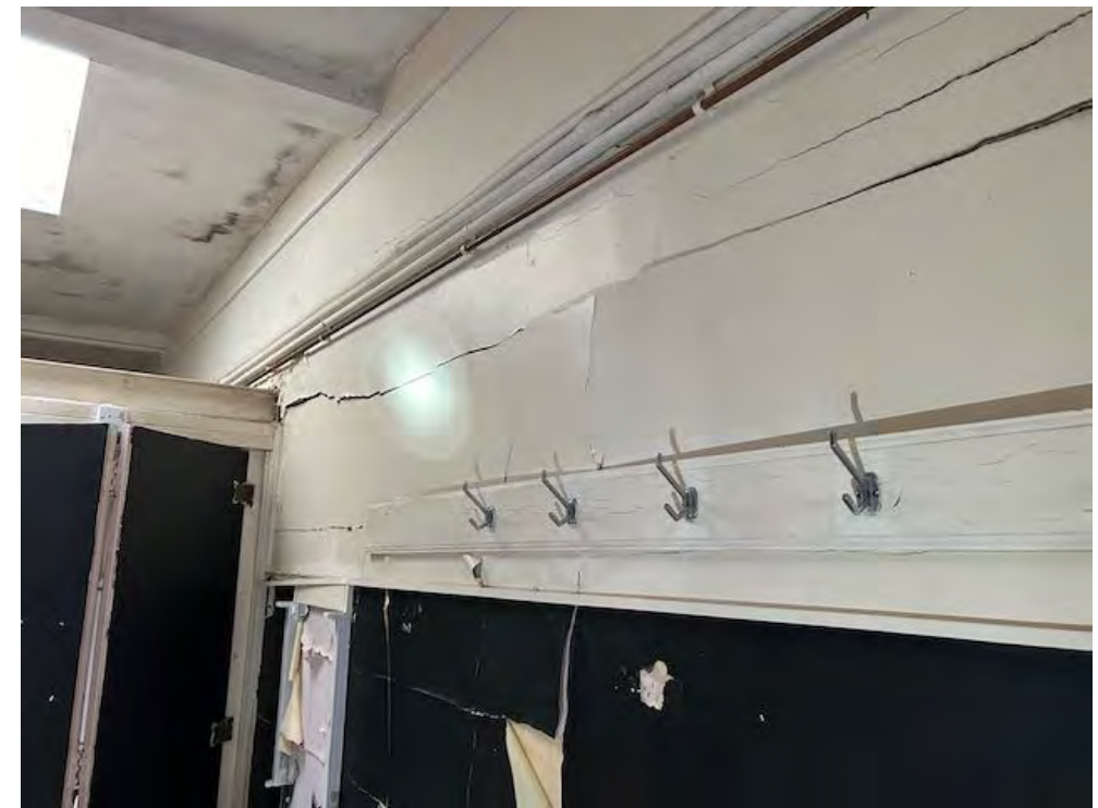
Horizontal cracking in wall due to failure of rib lath on damp south facing walls.
