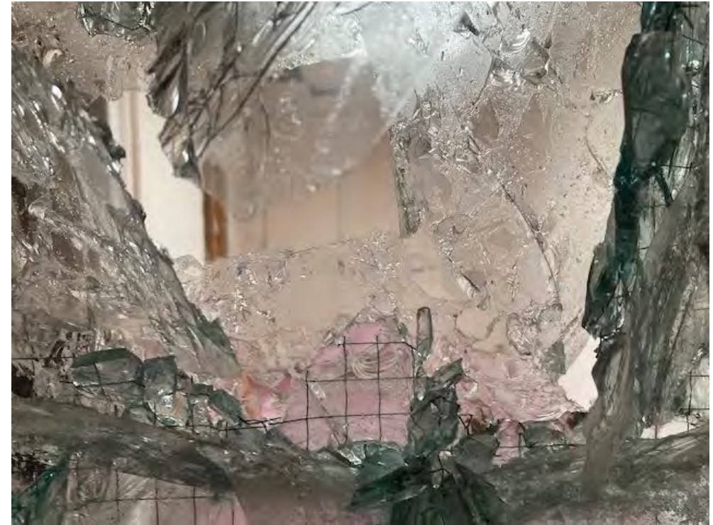
Broken door glass between office spaces in this area
