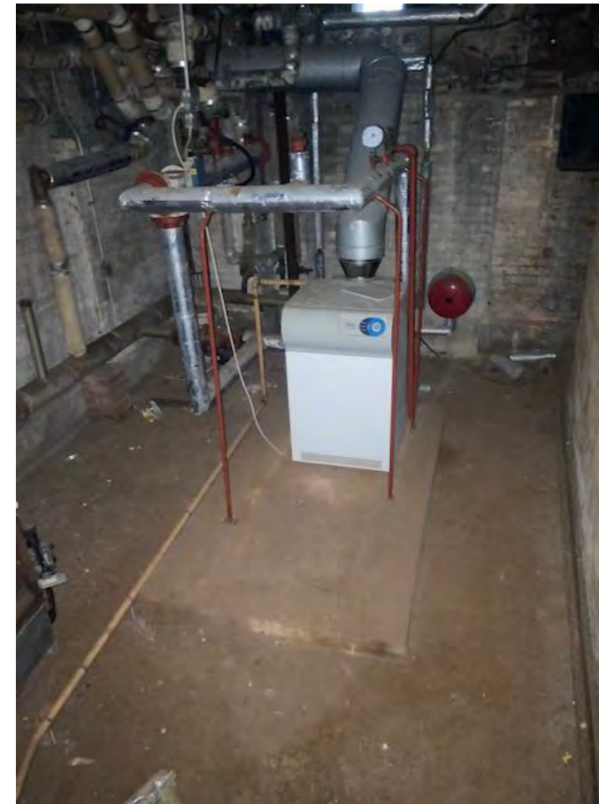
Oil (?) fired boiler in basement
