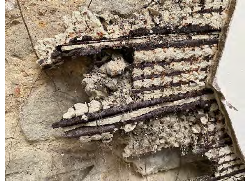
Corroded mesh within the plaster in the dressing rooms
