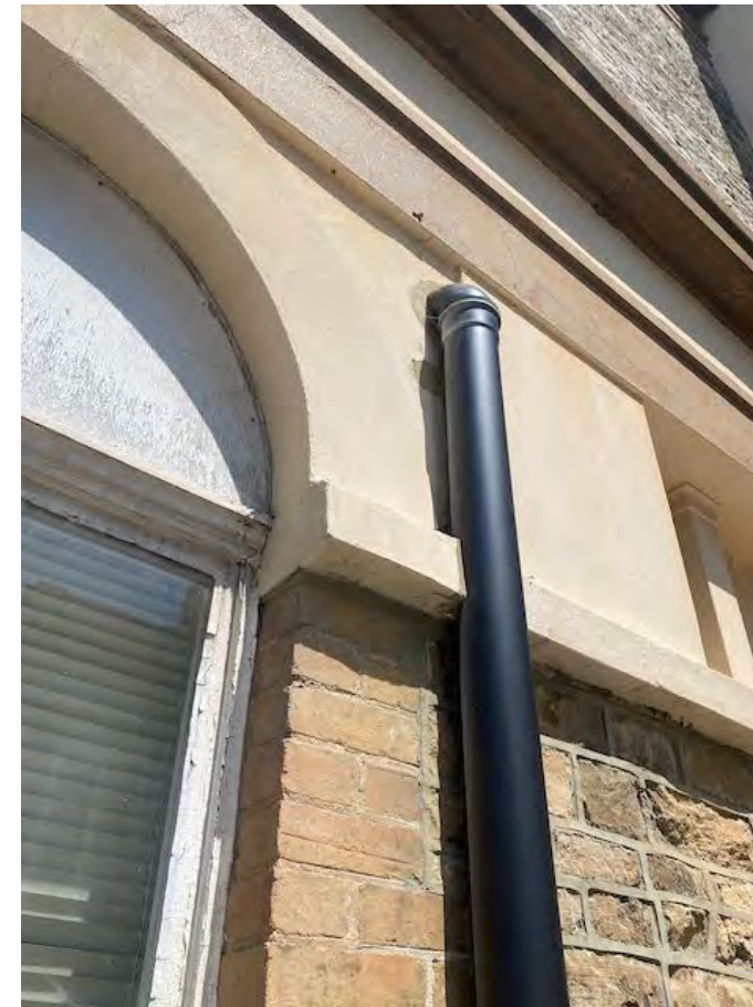
Rainwater pipe serving flat roof to west of main hall.
