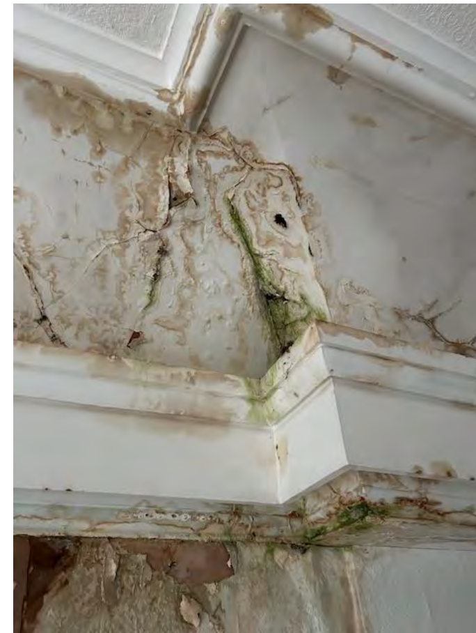
Active areas of damp below failing lead gutter. Very urgent repair required.
