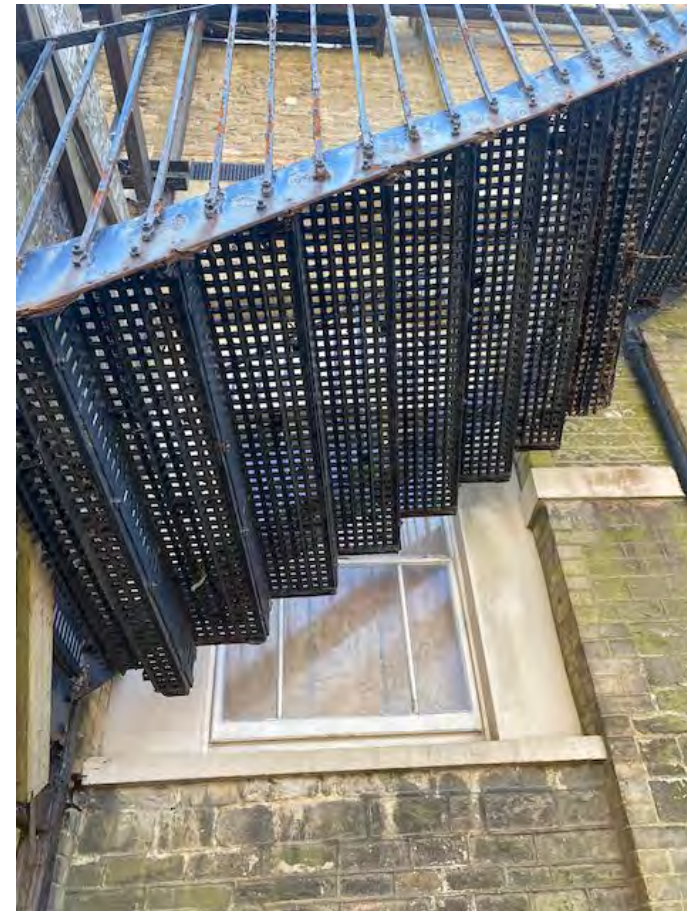
Damaged section of fire escape in imminent danger of falling (unsupported to inside edge). Urgent Work
