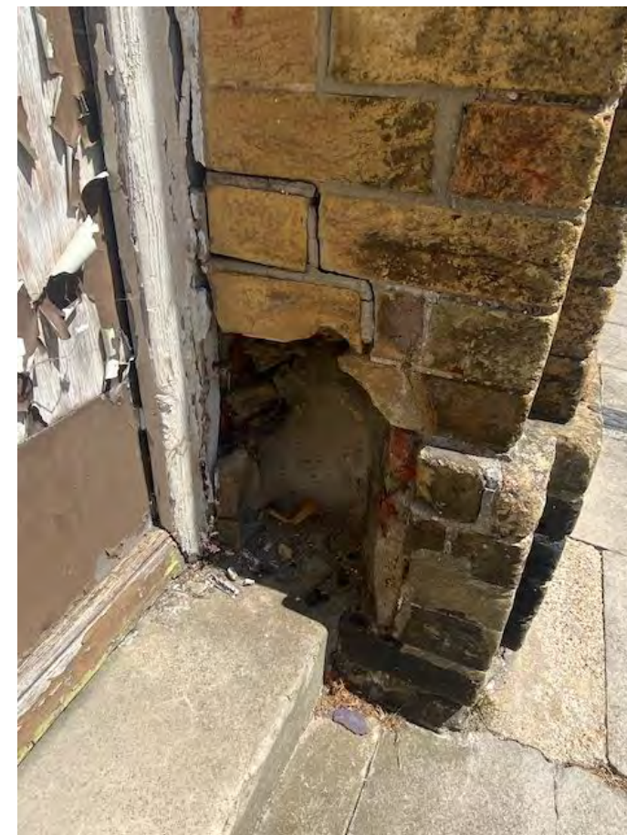
Area of damage next to door on the western pavilion
