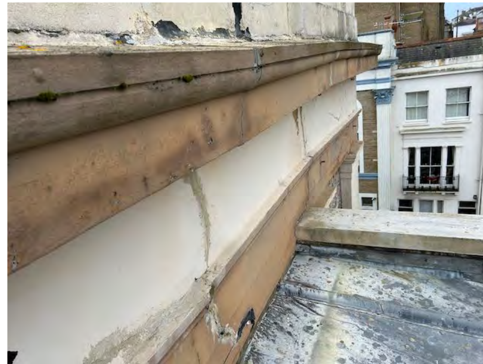
(Historic?) Movement below clock tower on West elevation visible in cornice.
