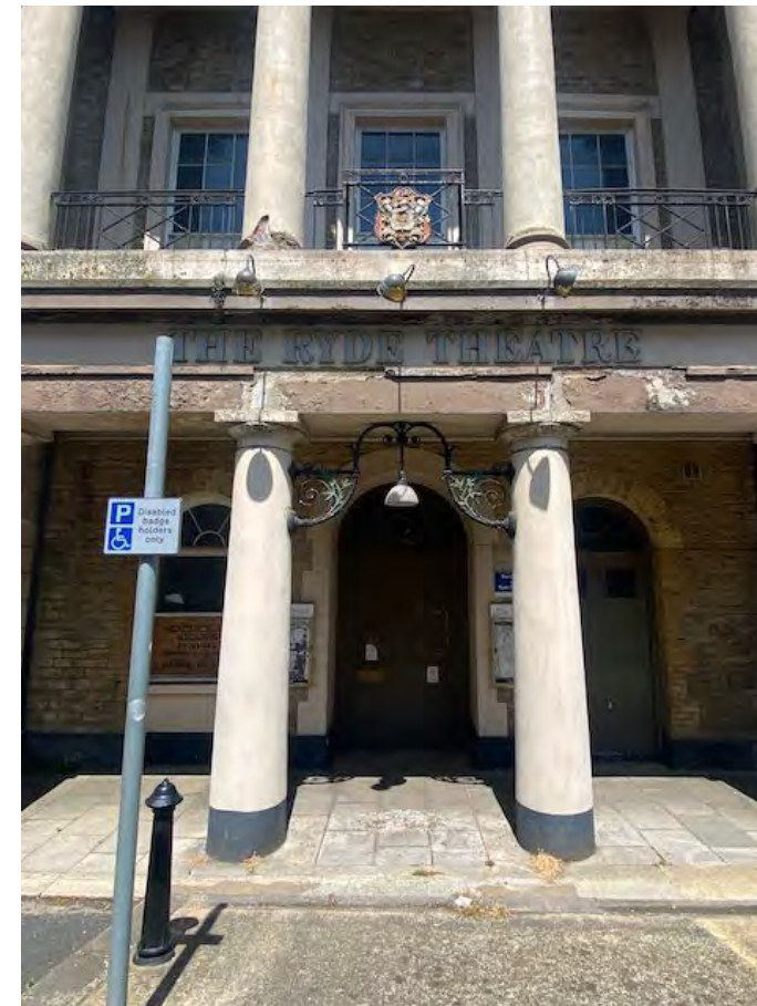
Stone lintel above the lower columns exhibiting blistered paint
