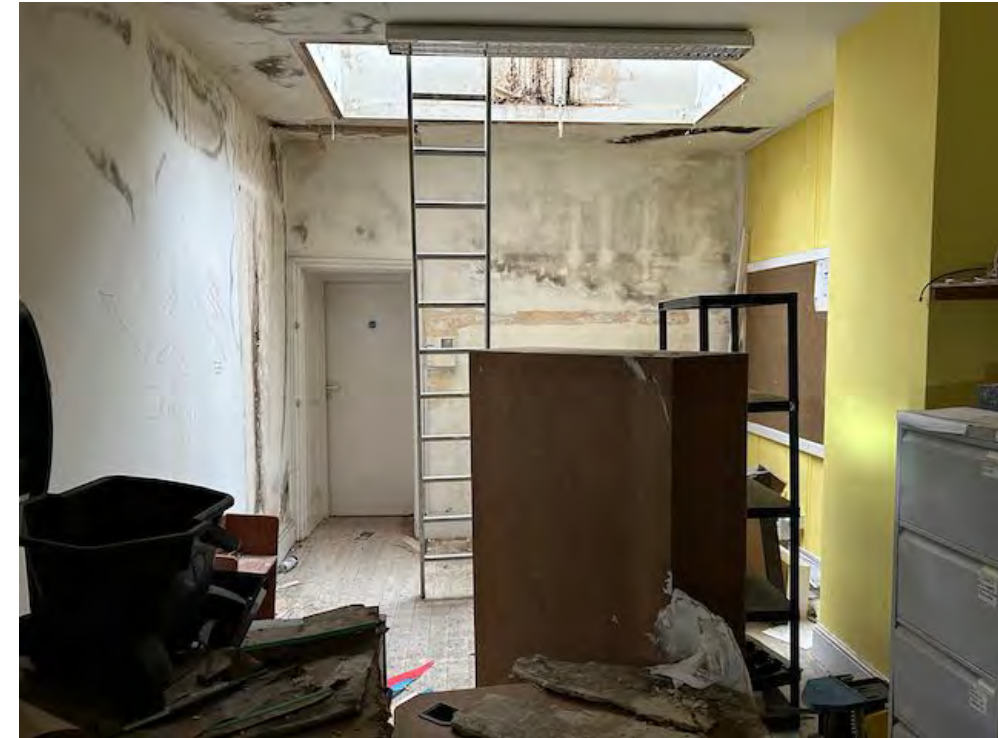
Upper office below clock tower. Note condensation where ceilings not insulated or ventilated.
