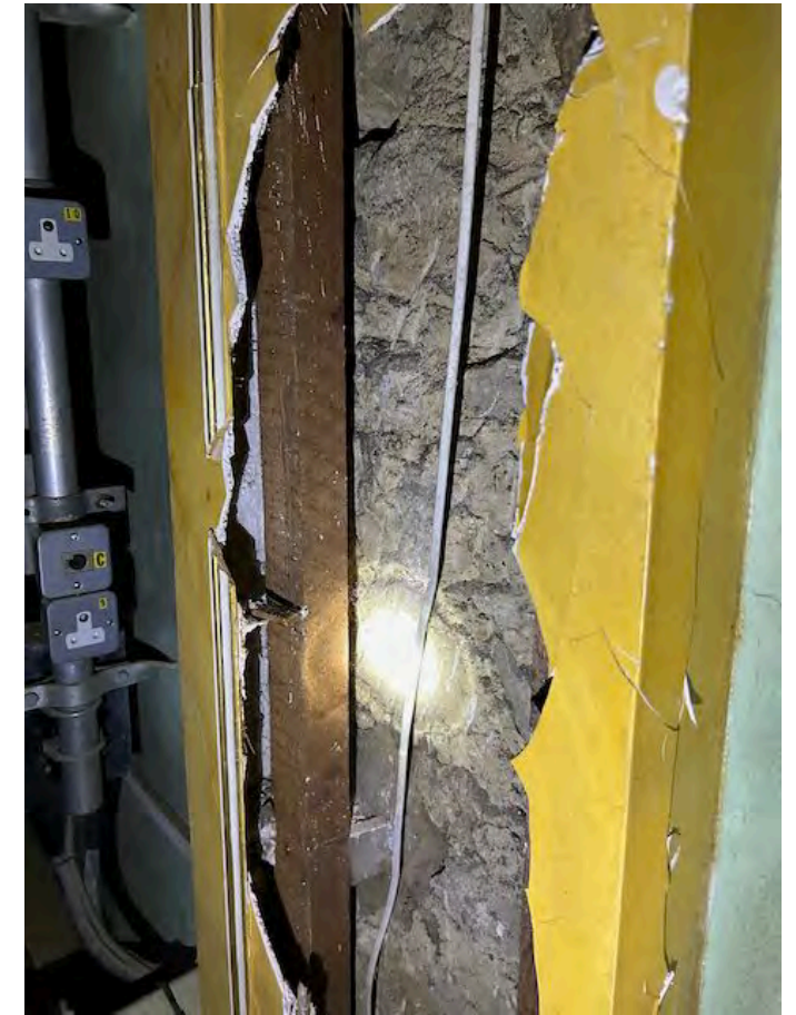
1930's timber grounds with hessian plastered finish over
