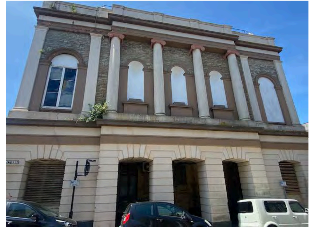
Buddleia growing on the South East corner of the building
