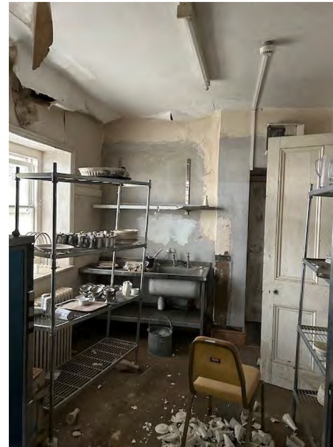
Vandalism in Ante Room
