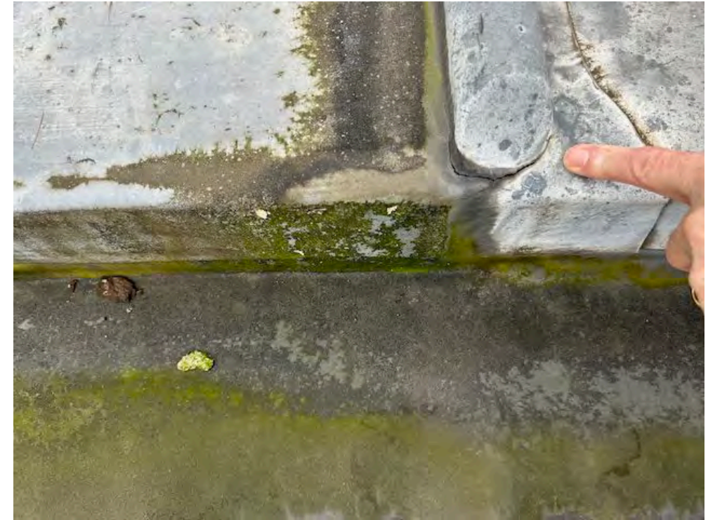
Overworked lead at the ends of each timber roll
