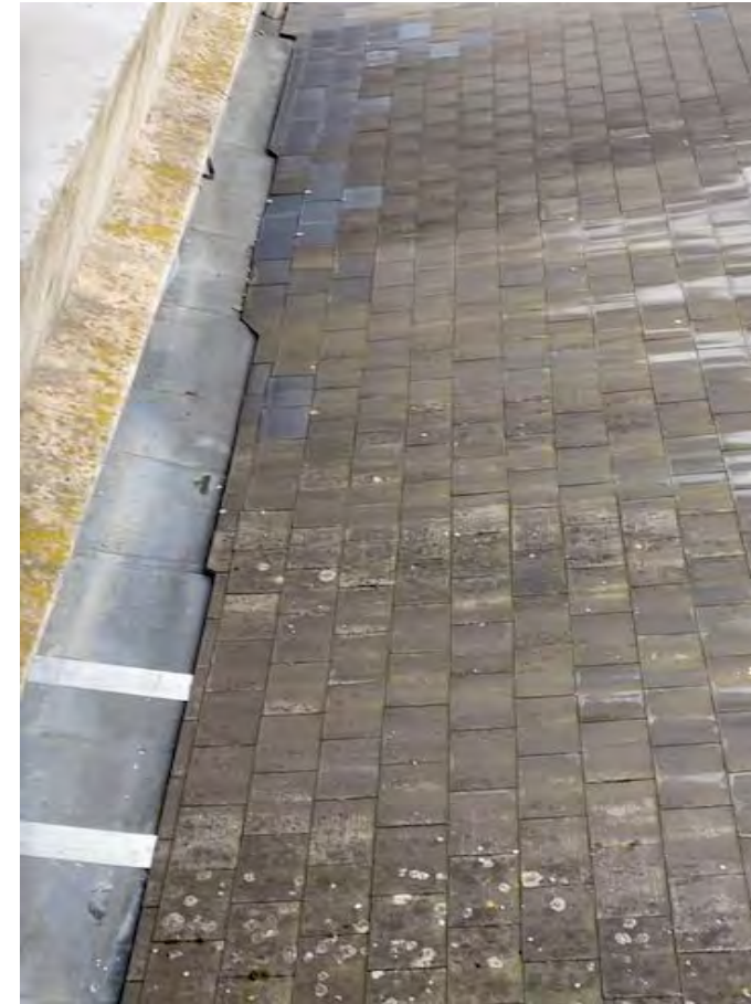
Lead lined gutter with Flashband repairs
