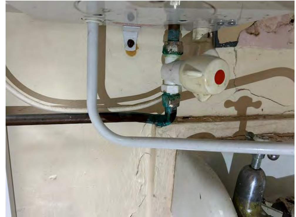
Leak below a sink in the changing rooms
