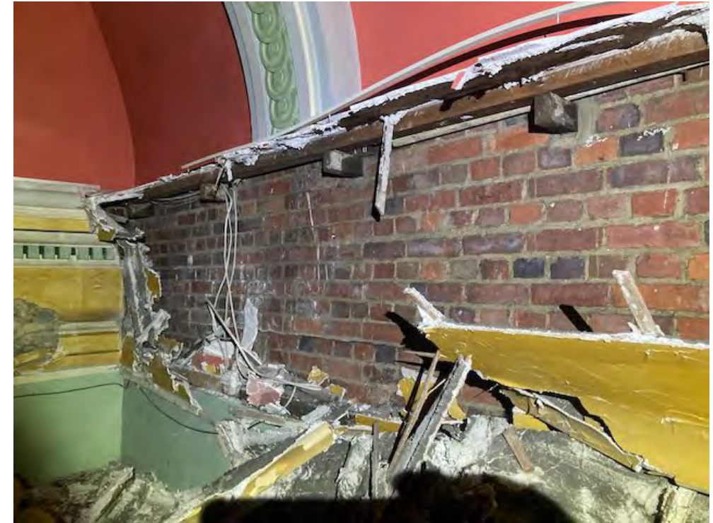
Damage to plaster coving on the north wall of the auditorium
