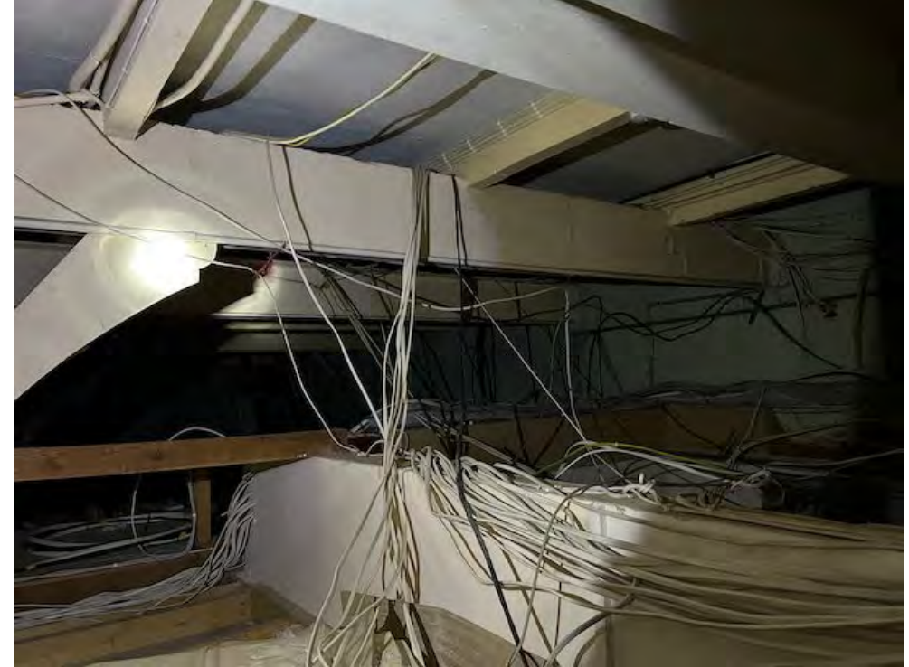
Vast quantities of wiring threaded through the building above the ceilings (East range)
