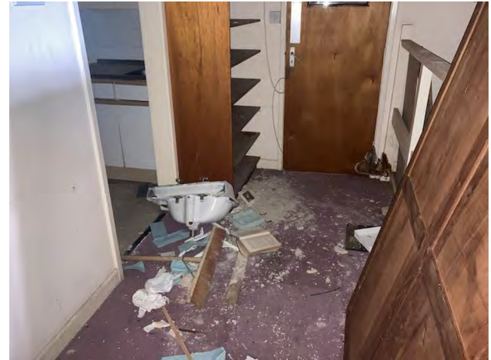
Dry rot fungus visible at bottom right of door. Vandalism.
