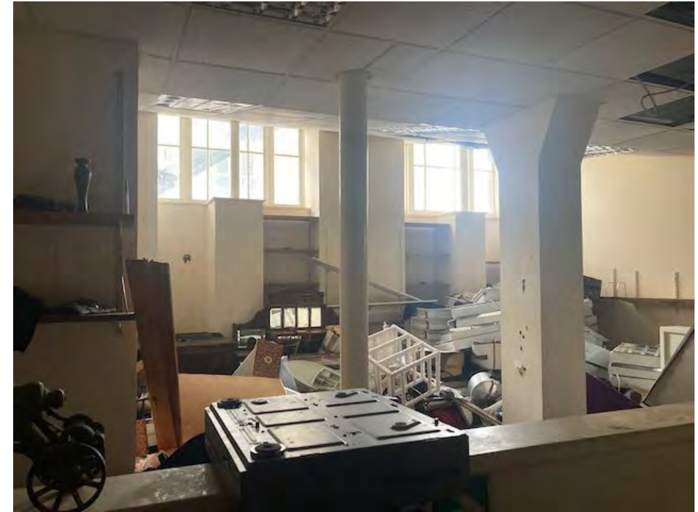
Modern debris to be removed
