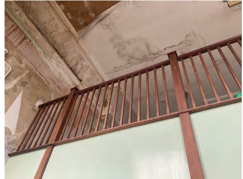
Damp penetration arising from spilt in lead lined gutter above (See pp17).
